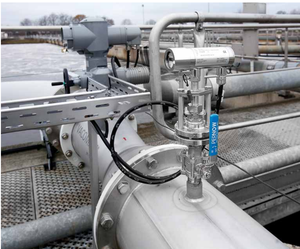
The left top photo shows the installation of the VACOMASS® flow meter SS in combination with the torsion-proof hot tapping unit OEIN-F. The right top photo shows the VACOMASS® flow meter AL 100 with the integrated simultaneous flow profile compensation of the flow signal.
